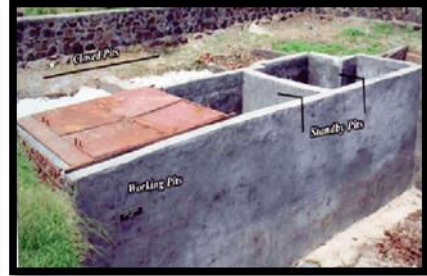
Deep Burial facility
